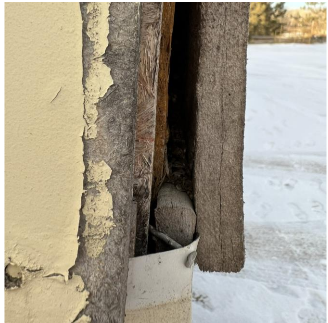
Missing corner flashing exposing fibrous siding ends & sheathing
