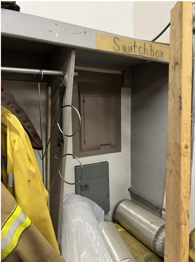
Electrical panel with insufficient clearances
