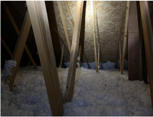
Maintenance area attic space was inspected, and the roof sheathing appears to be in good condition. The soffit baffles are properly installed, and the blown-in insulation is evenly distributed
