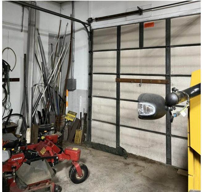
Water staining at the base of the overhead door indicates water pooling in the area.
