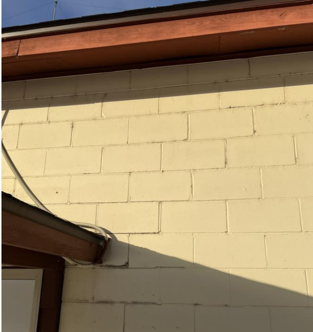
Instance of stair-step cracking near entrance
