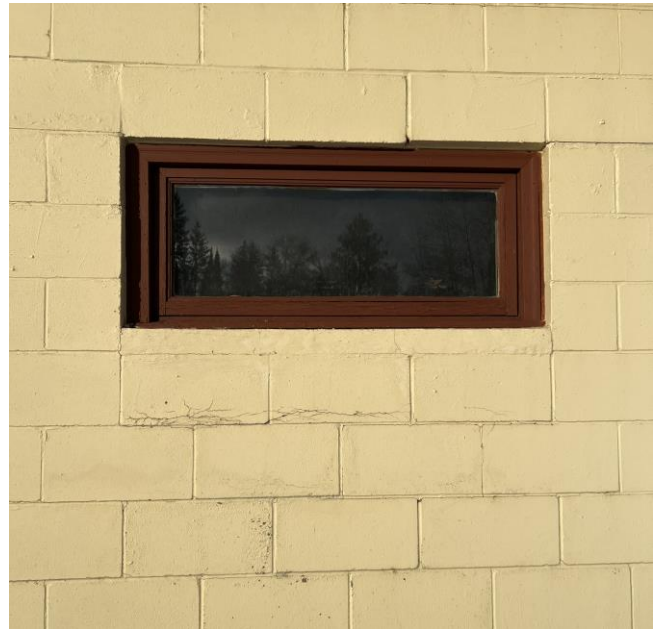
Instance of CMU spider cracking beneath wood awning window
