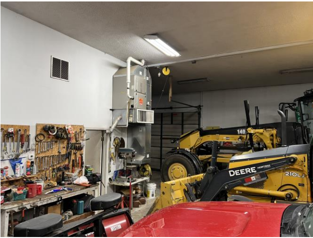
Maintenance area mechanical unit
