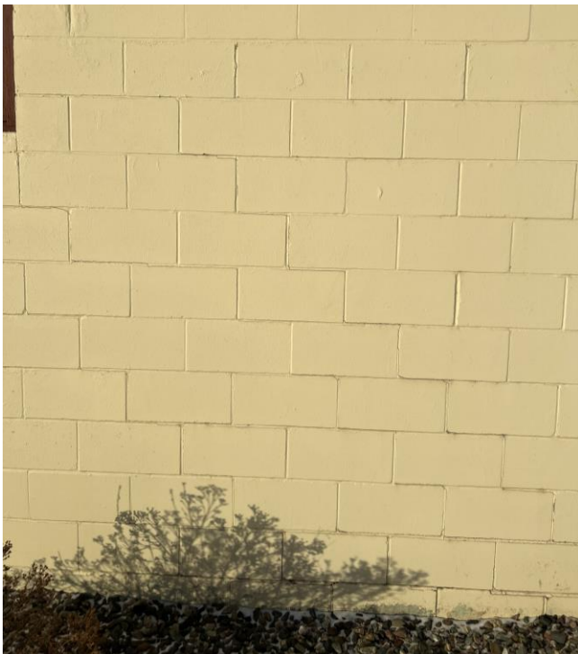
Instance of stair-step cracking in south wall
