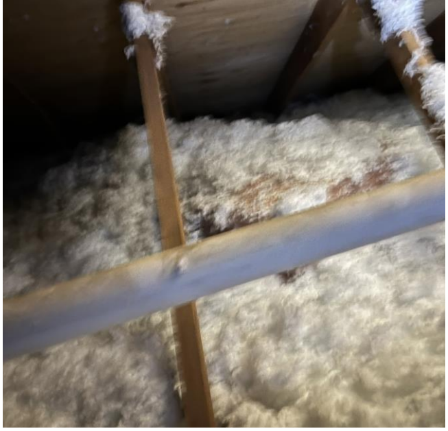
Blown-in insulation compacted at soffit with no evidence of baffles
