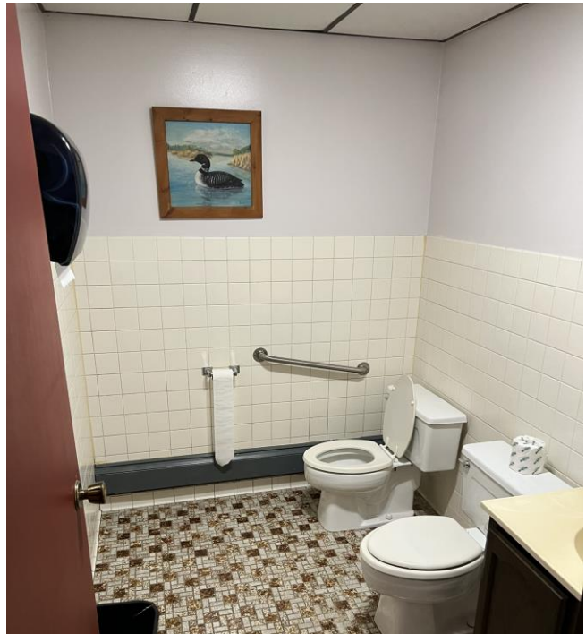
Lack of privacy in women's restroom
