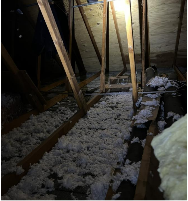
No insulation at adjoining roof structure
