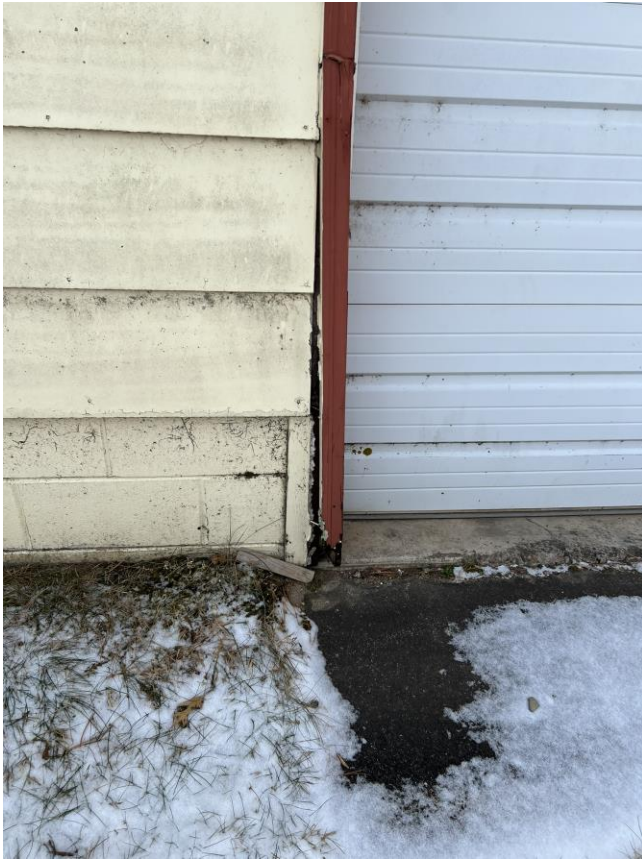
Wood door jamb separating from structure
