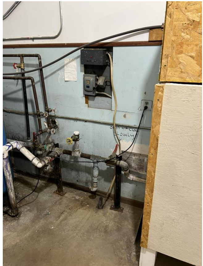
Controls and piping for pump that no longer believed to be in service. Loose Romex wire should be properly protected.
