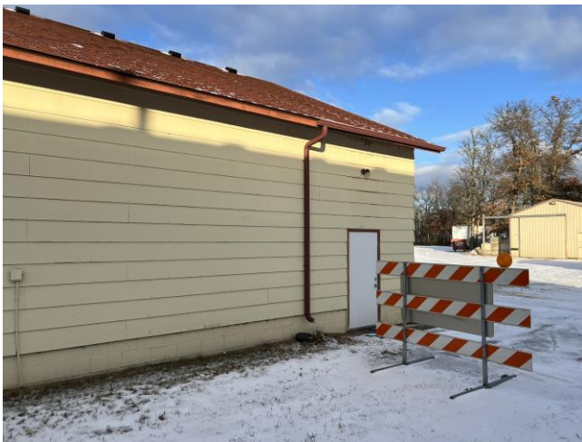
Down spout with missing diverter
